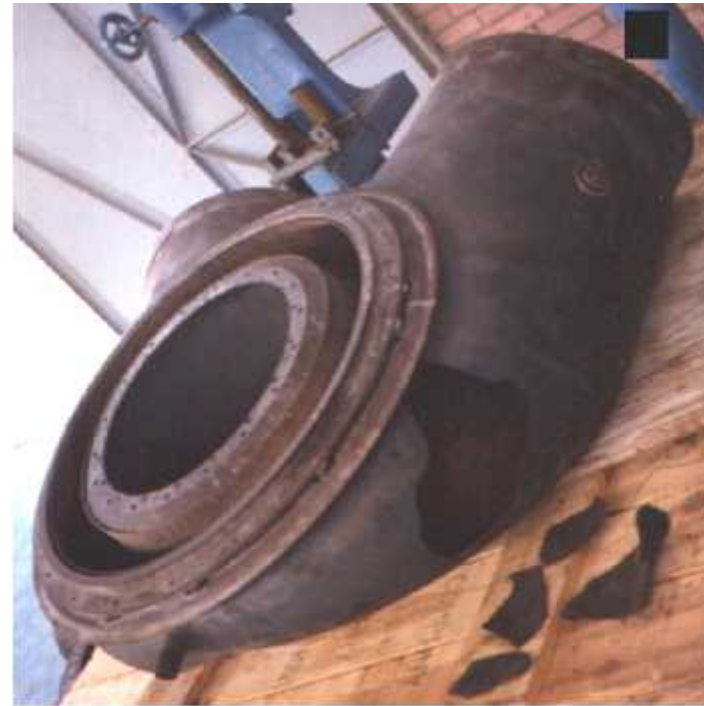
Gas Duct at GUPCO Power Station
