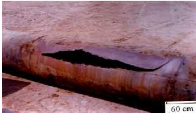
Line SUMED Pipe
